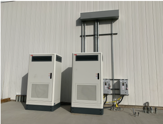
Photo: UMass External EV Bus Charger Units in Place
